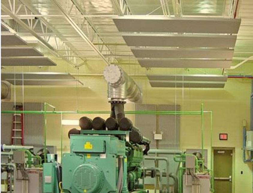
Cloud Panels In Mechanical Room
