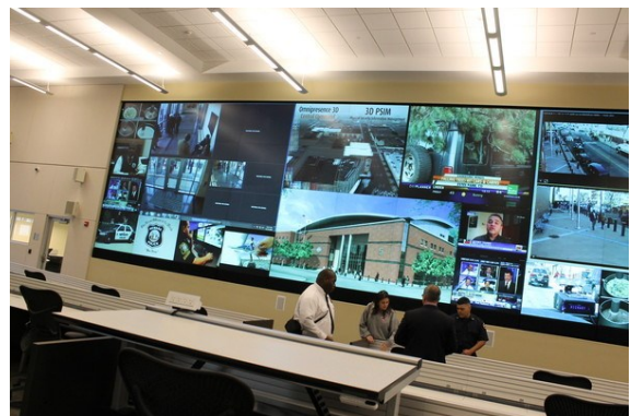
Command Center monitors city video feeds
