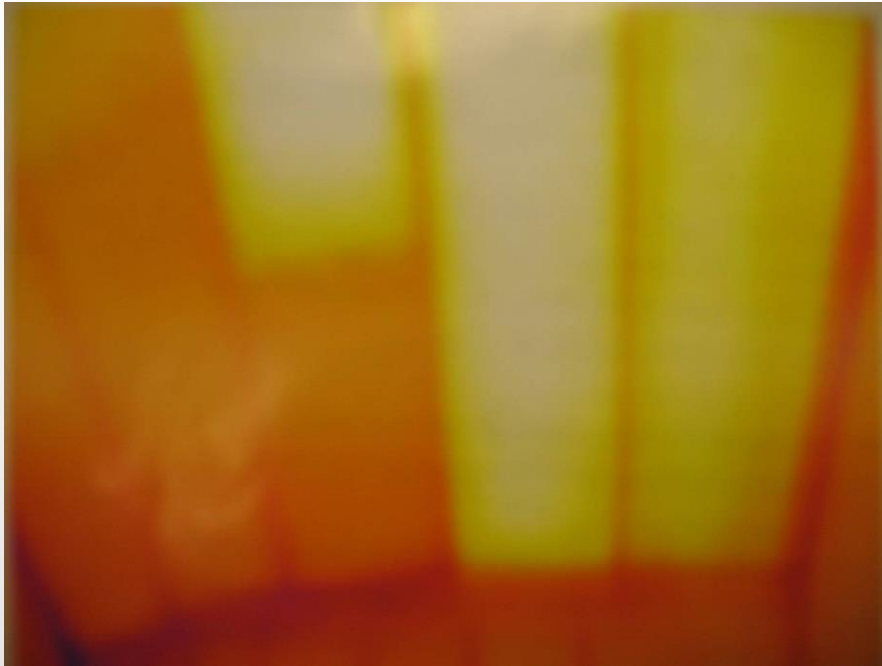
Missing Ceiling Insulation
