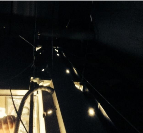
Hot and cold air readily passes through the steel housing and fixture holes
