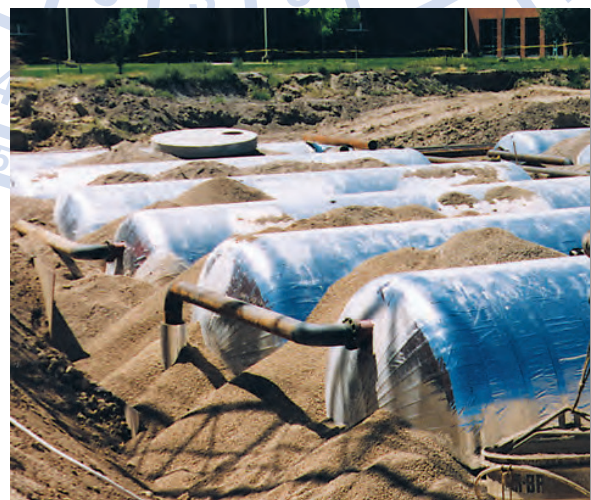
These buried hot and chilled water tanks were insulated with Pamrod HATS for trouble-free performance.
