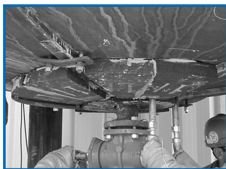
Vessel heads with heat tracing lines present an insulation challenge that can be overcome with Pamrod HATS.
